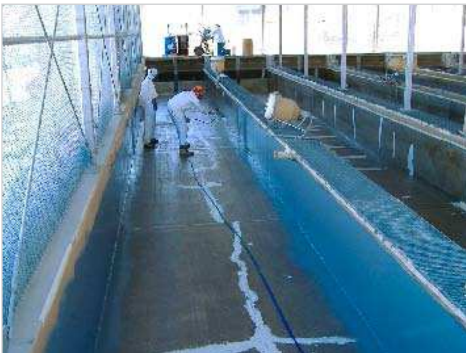
Contractors applying an environmentally safe coating in an LCT runway at Lahontan NFH.
